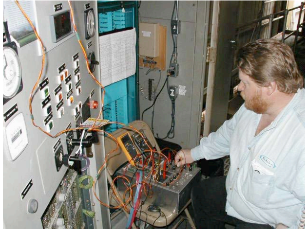
Bill Fish simulates turbine operation using the Calibrator
