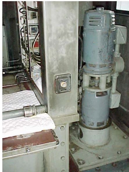
Fig. 1: Emergency Lube Oil Pump and Motor (motor on top, 88QE)
