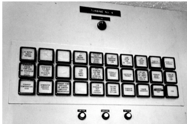
Fig. 6: Low Lube Oil Pressure Alarm, (Second Row, 8 th from the left, Drop #18 here)
