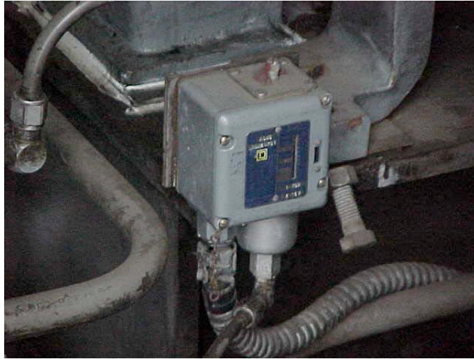
Fig. 4: Lube Oil Pressure Switch Trip, 63QT, Located at Generator Pedestal
