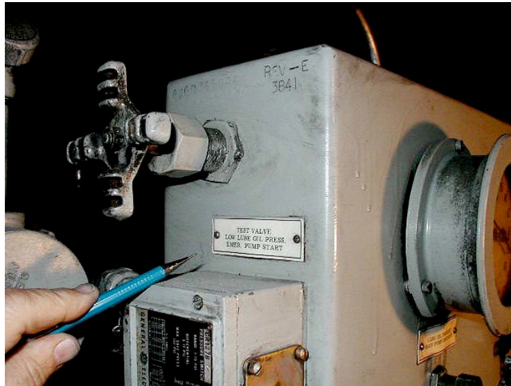
Fig. 5: Test Valve for Low Lube Oil Pressure – Emergency Pump Start
