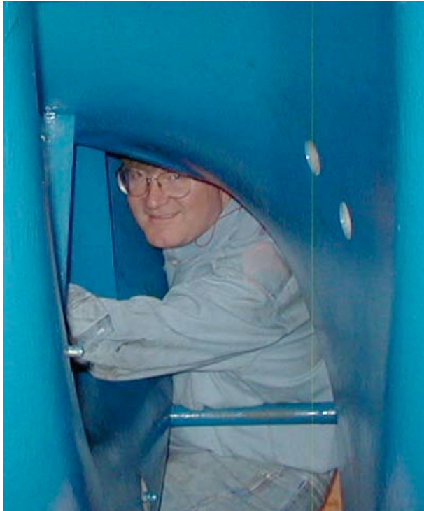
Charlie Pond setting IGV angles inside inlet bellmouth of MS6001B gas turbine
