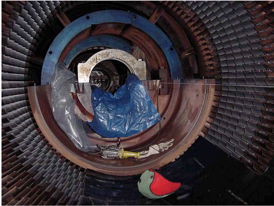
Wire running through the compressor, inner barrel lower half and #2 bearing on a Frame 7E
