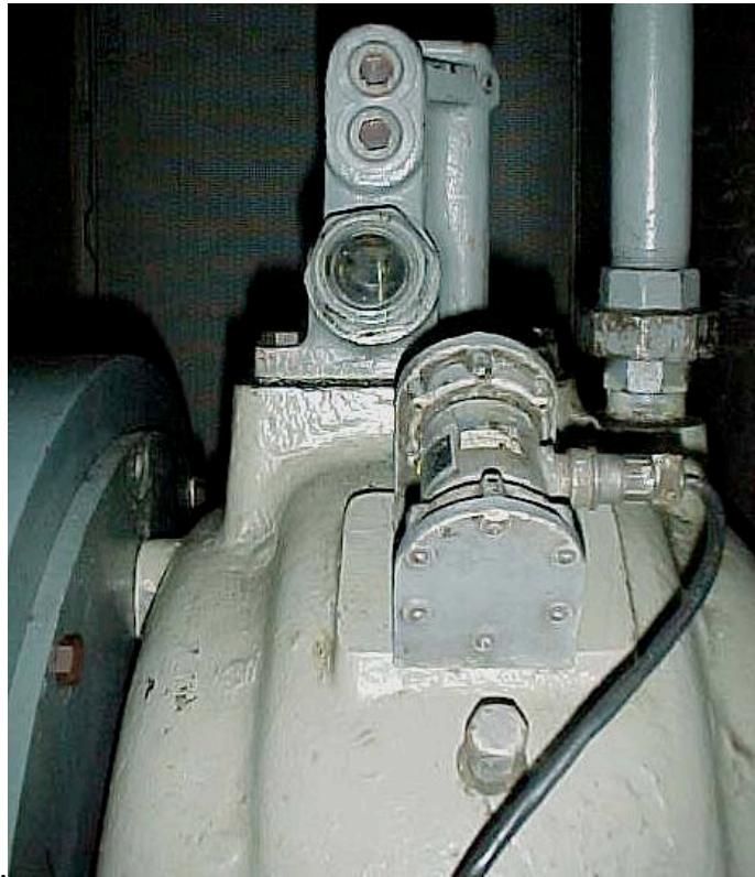
Fig. 3: Vibration Detector mounted “side saddle” on a Generator Bearing Pedestal
