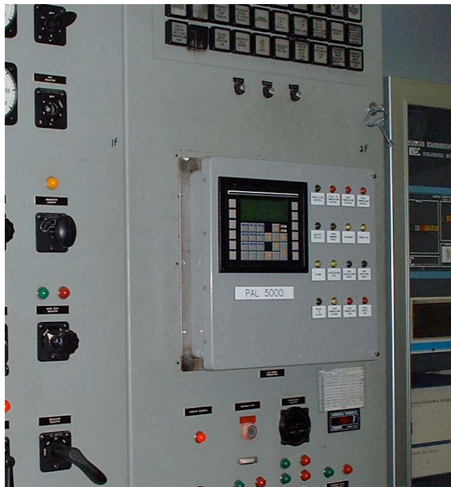
Fig. 3: PAL 5000 Control & Protection System at Liberal, KS
