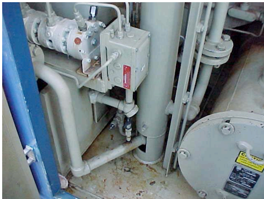
Fig. 4: HP Filter and Flow Divider with associated piping
