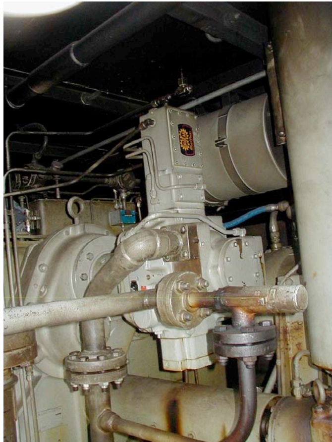
Fig. 1: Typical OilGear Fuel Pump on MS5001LA gas turbine
