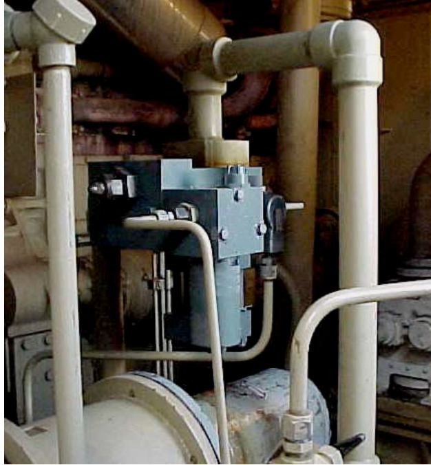
Fig.4: Fuel piping inlet leading to the Bypass Valve (blue, center)
