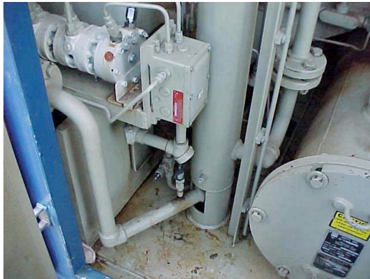
Fig. 3: HP Filter (vertical) and fuel oil pipe leading to Flowdivider
