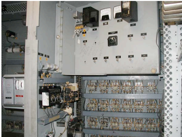
Fig. 1: GE control panel with Ward-Leonard relays on rear wall
