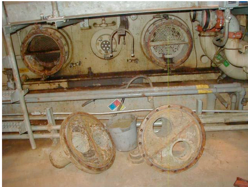
Fig. 3: Lube Oil Heat Exchanger (Cooler) Covers
