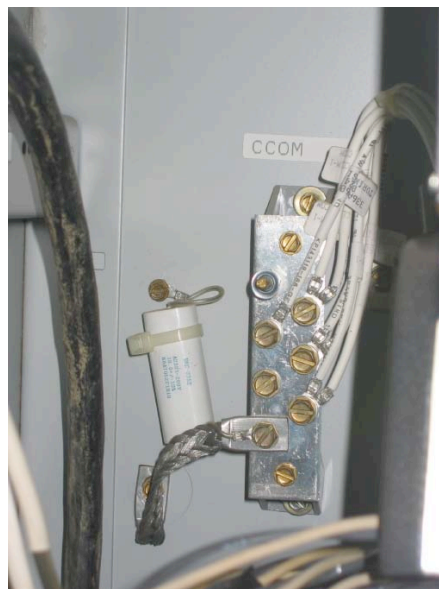
Photo of Ground Strap
