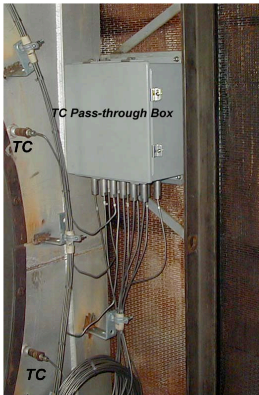
Fig. 3: Thermocouple connections under the inside "pass through" box
