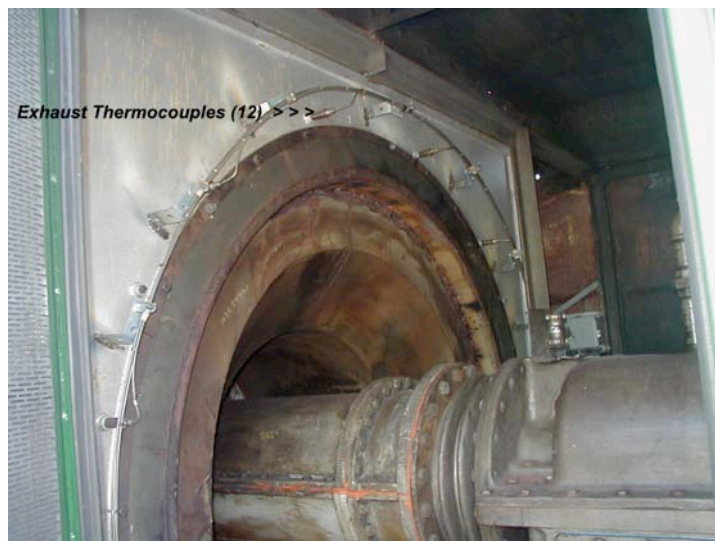
Fig. 1: Exhaust thermocouples encircle gas turbine exhaust plenum
