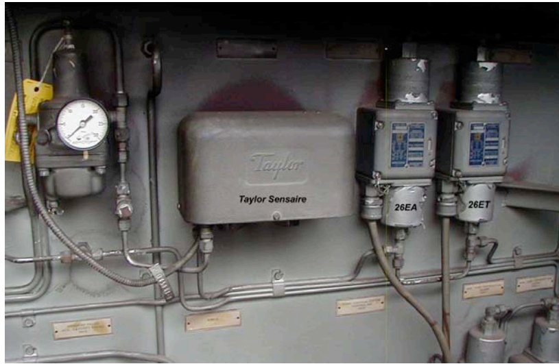
Fig. 2: Taylor Sensaire – Compressor Inlet for Ambient Compensation
