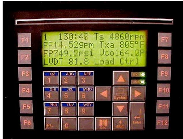
Fig. 5: PAL5000™ Protection System showing Exhaust Temperature, Txa
