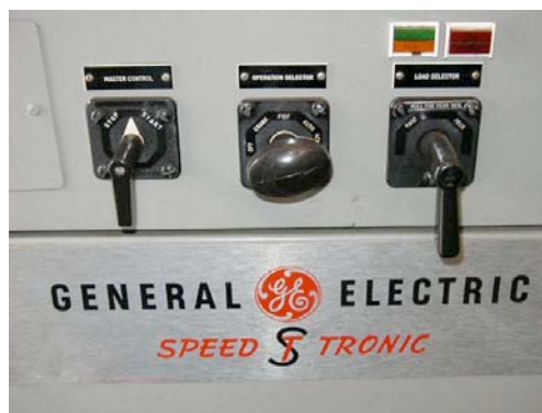
Fig. 1: Operation Selector Switch in Remote Start Position at Base Load
