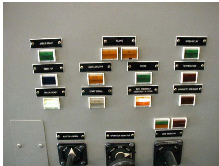
Fig. 6: Panel Lights (speed relays, flame detection, fuel controls)
