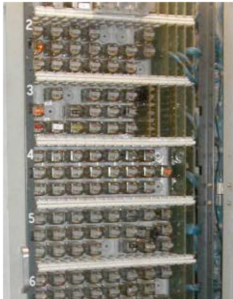
Fig. 3: Typical MS7001B Control Panel with over 100 relays
