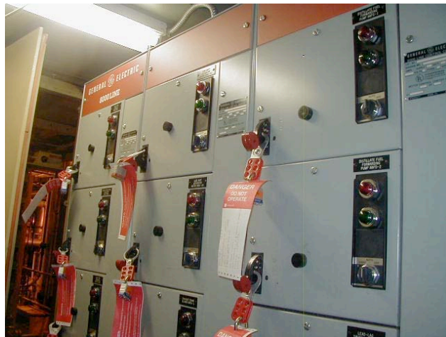
Fig. 3: Motor Control Center (MCC) showing switch in the upright AUTO mode (lower right side)
