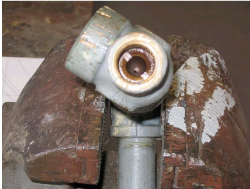
Fig. 3: Cover removed on venturi, opening clogged
