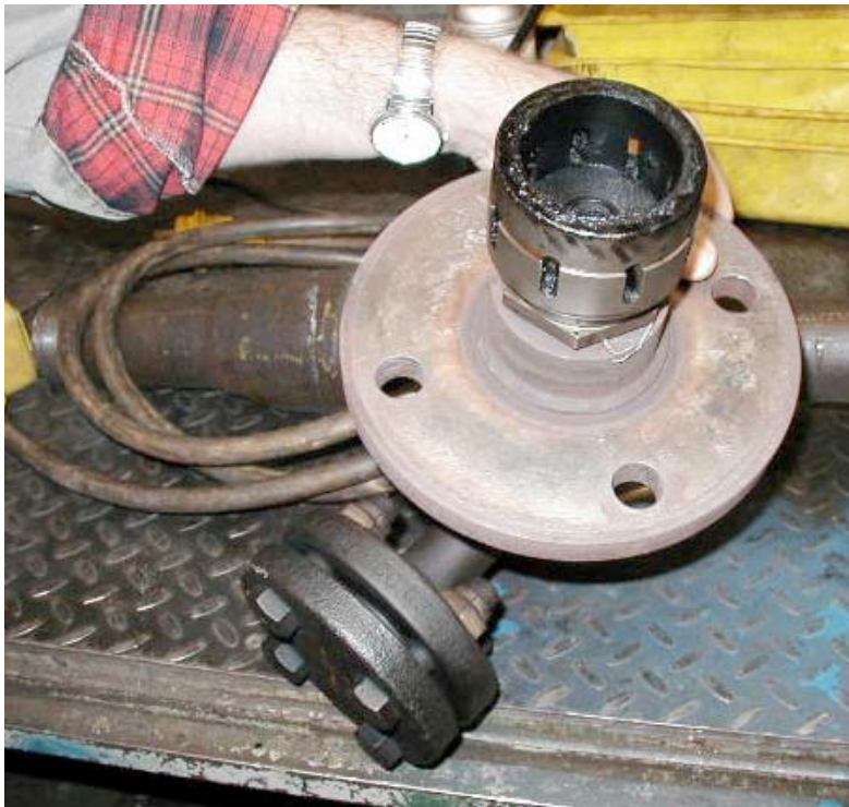
Fig. 3: Coked up RVG Liquid Fuel Nozzle (as viewed from discharge end)
