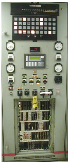
Fig. 1: Typical Speedtronic™ Control Panel with lower door removed
