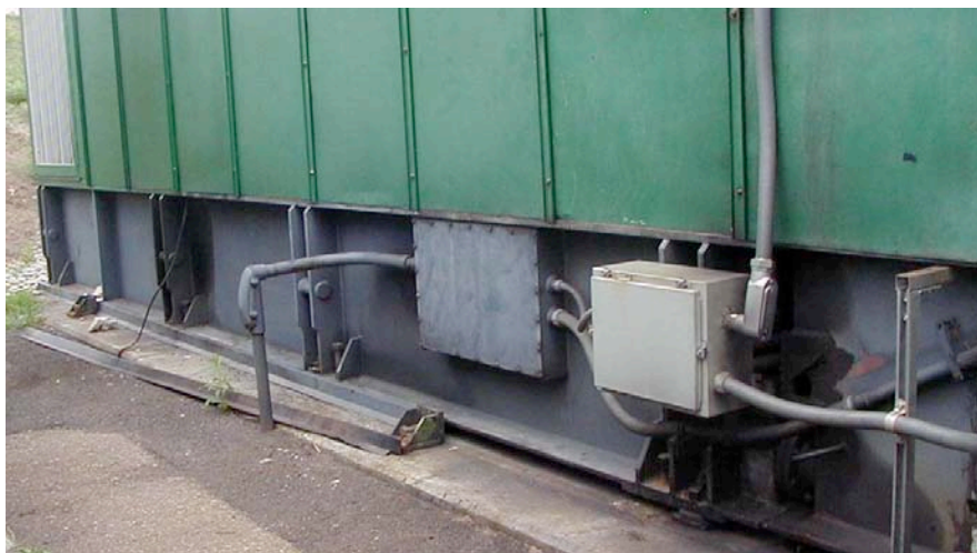
Fig. 1 – Original JB and New Pull-through Box and Conduit for “Home-Run” Wiring
