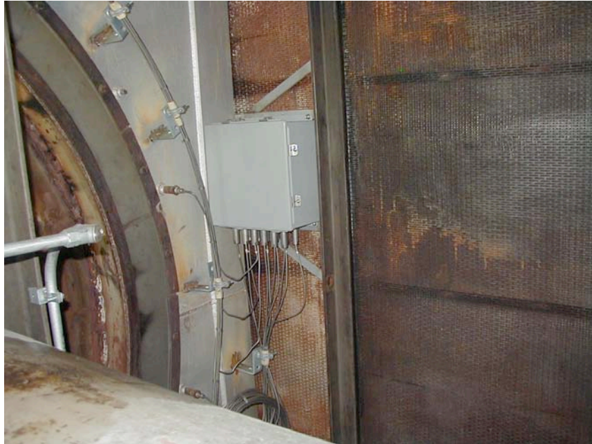
Fig. 2: Pull Boxes, Conduit and New Thermocouples “home run” to Control Room
