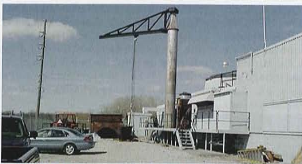
1. MDU's Frame 3 gas turbine in Williston, ND, is still operating after more than 50 years on the job
