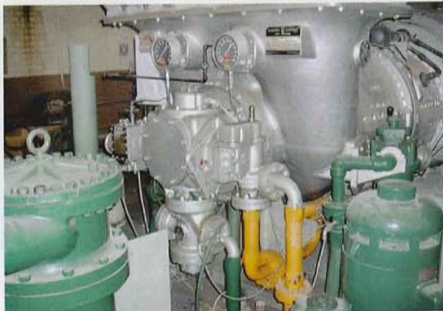
5. Gas-only machine. Fuel gas controls (orange piping) are at the front of the axial compressor. Note the stop valve hanging off the gearbox. Accessory base for a gas-
