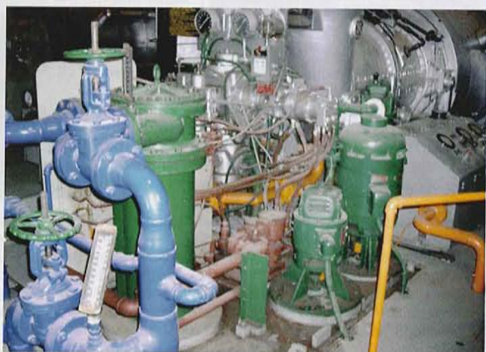
3. Motor-driven auxiliary pumps, filters, valves, etc., are located on the accessory base. Liquid fuel system is in the center with all the hoses (right)
