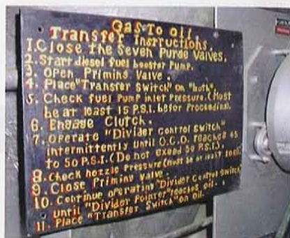
7. Instructions remind operators how to transfer from gas to oil during operation
