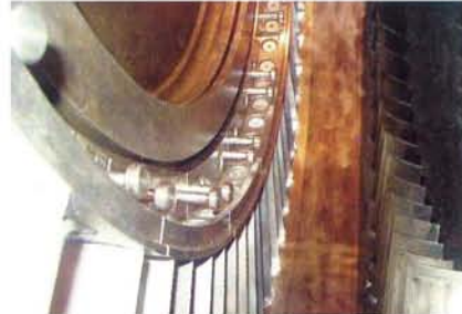
8. T pins replace original dowels in the lower half of the bellmouth to facilitate access to guide vanes in future outages
