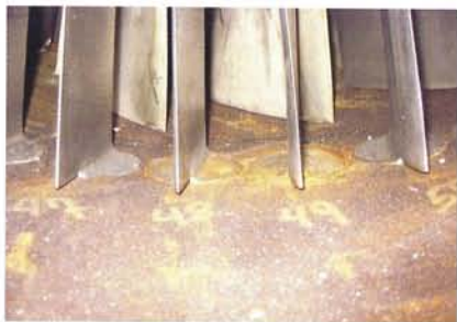
2. Vanes 48 and 49 are in the 6 o'clock position and the ones most likely to have corroded thrust washers
