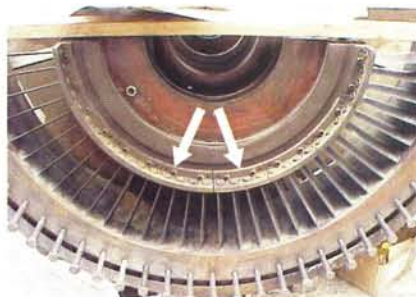
5. Inner ring segments are in evidence on lower half of bellmouth from unit where the shaft was removed
